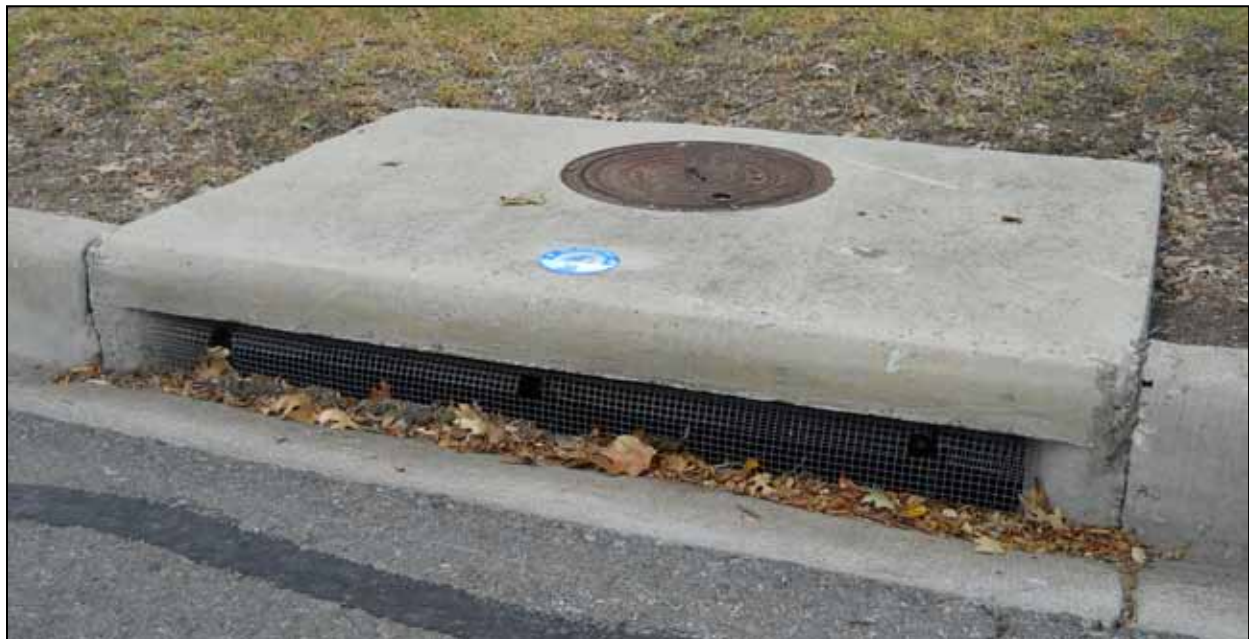
Figure 6. Lockhart storm drain inlet protection and storm drain marker.
